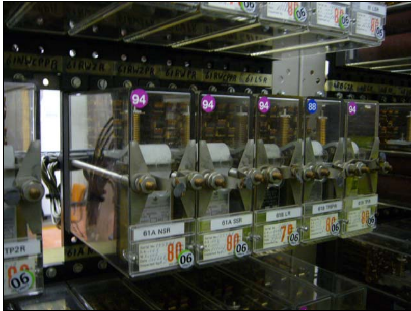
Photo 3: A close up of a bank of relays.
