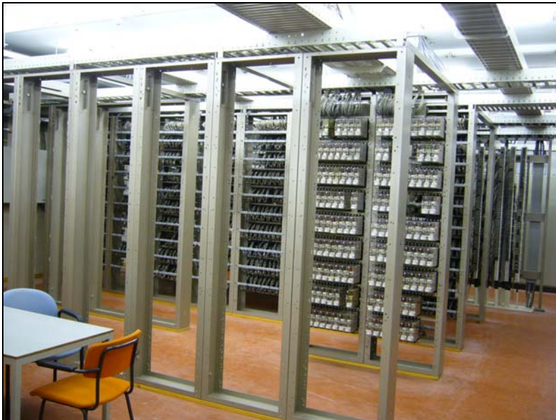
Photo 2: The relay room at Swolle Station.
