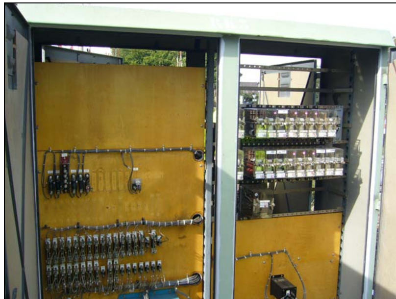
Photo 6: The relay cabinet that controls the level crossing.
